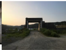
Former levee passage left after being partially destroyed *as of August 2015
